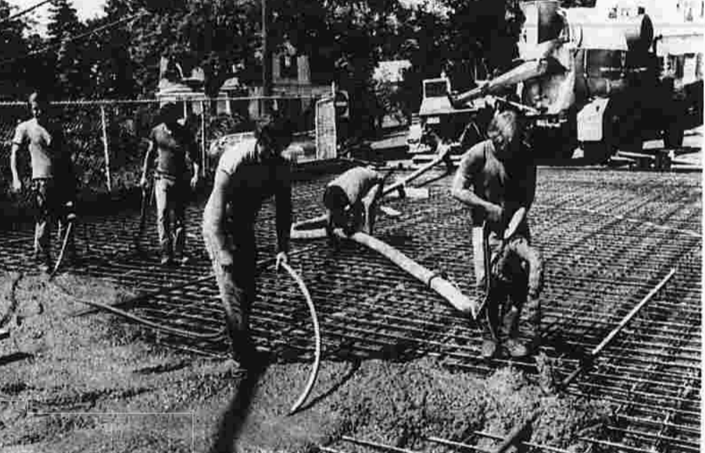
New Bridge Is Born When a new bridge is born, everyone gets in on the act. Workers from the Black and Warner Construction Co. use a vibrator and cement mixer to spread out the concrete at the site. (Herald photo by Pinto)
